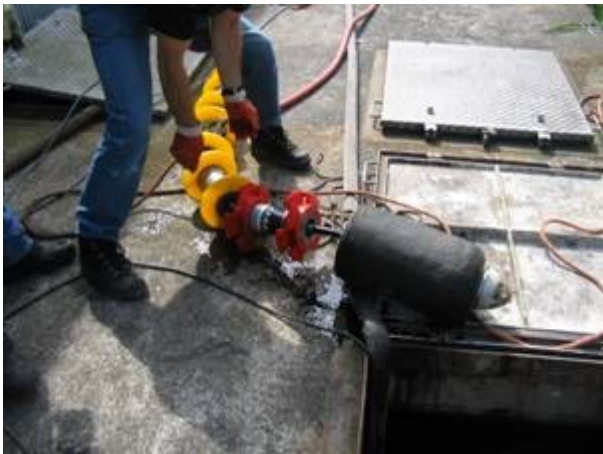
Inspection pig as used for the inspection of the HDPE sewage pipeline
