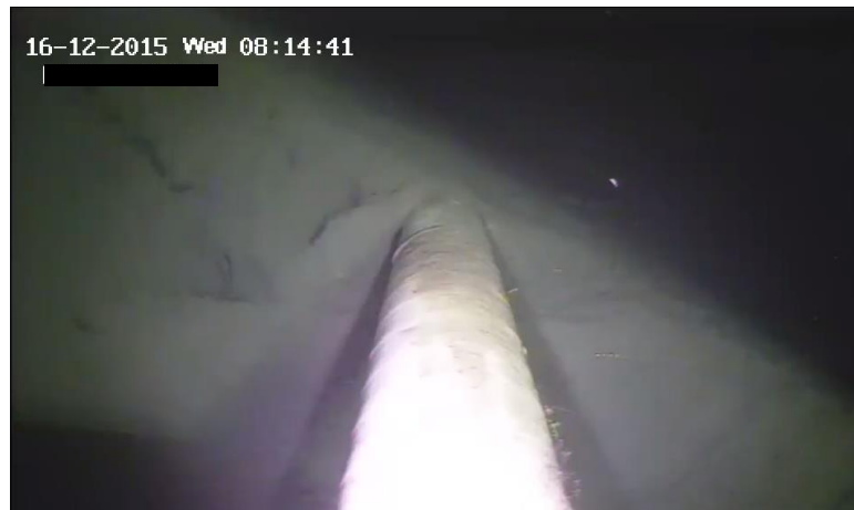
Figure 12: View of the pipe and the seabed after intervention. The picture is taken from the camera on the crawler.
