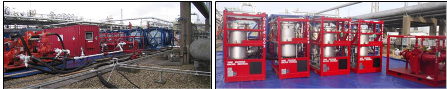
Onshore Receiving and Pumping Spread at Terminal
