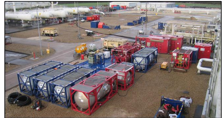
36" X 118.7km Gas Export Flushing Station
