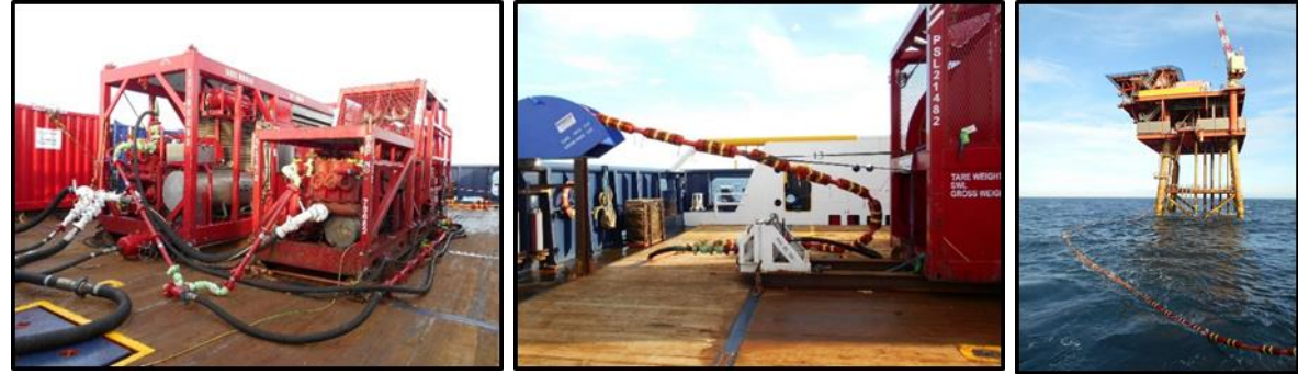
Supply Vessel Based Flushing Spread c/w Flushing 2" HP Hose Deployed to Satellite
